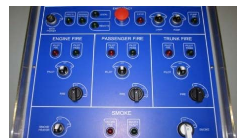
control panel control of the fires and smoke
